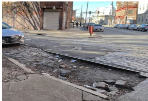
Figure: Example of potholes and cracks: Callowhill Street (Source: Authors, 2022)
