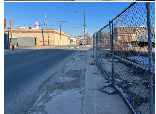
Figure: Fading crossings and broken sidewalks (Source: Authors, 2022)
